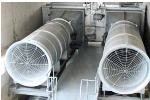
Station and tunnel ventilation equipment
