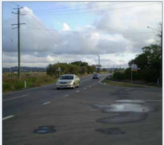
Bottom right: Image looking west along David Low Way from the David Low Way/Finland Road intersection
