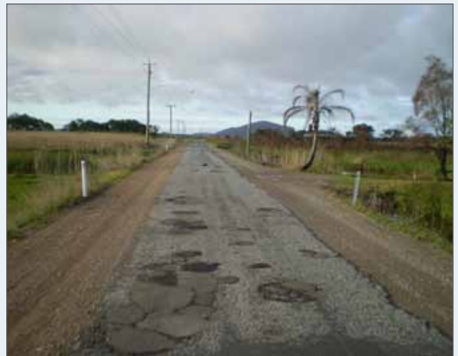
Top right: Image looking north along Finland Road, showing poor pavement condition (first section) and flood susceptibility
