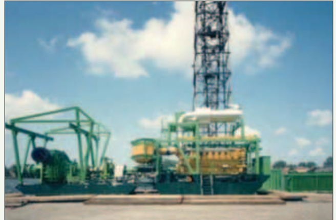
Figure 5.4m: A booster station during the establishment stage. The pump and engine are mounted on two skid pads
