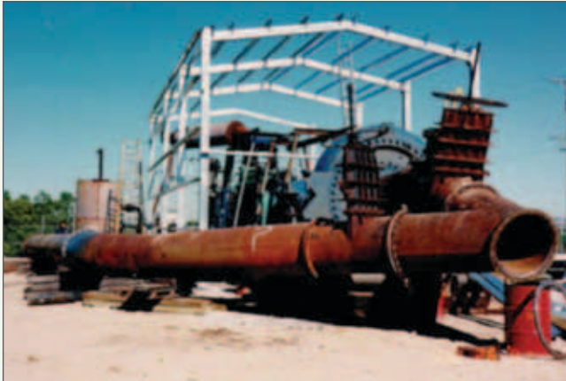
Figure 5.4l: Booster pump station under construction. Photo shows bypass line, valve set, sand pump and frame for housing
