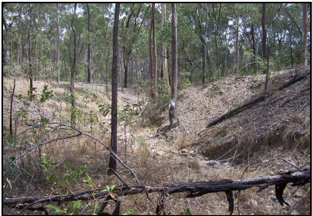
Photo 2 Evidence of erosion in the upper part of water course (flowing to the south)
