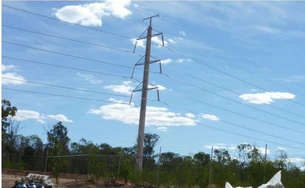
Figure 3.15.2 132 kV Power lines
