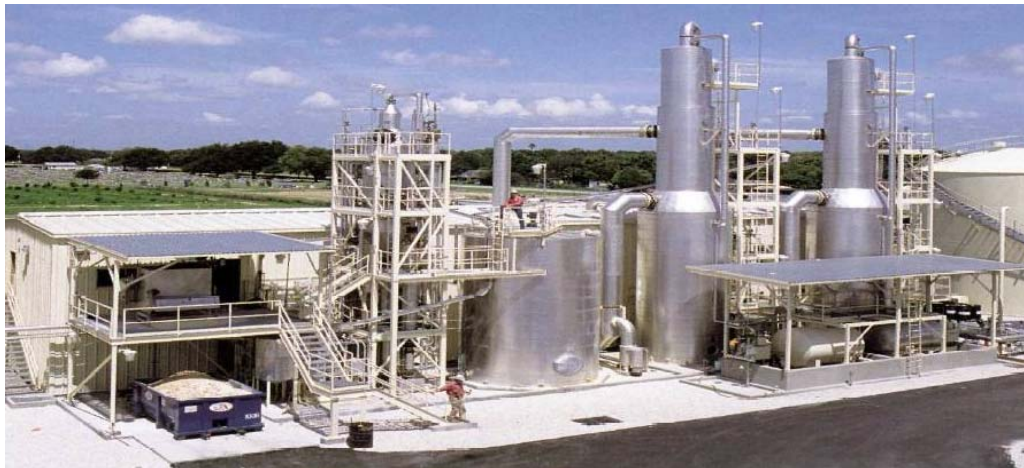
Figure 3.15.3 Water Treatment Plant with Brine Concentrator
