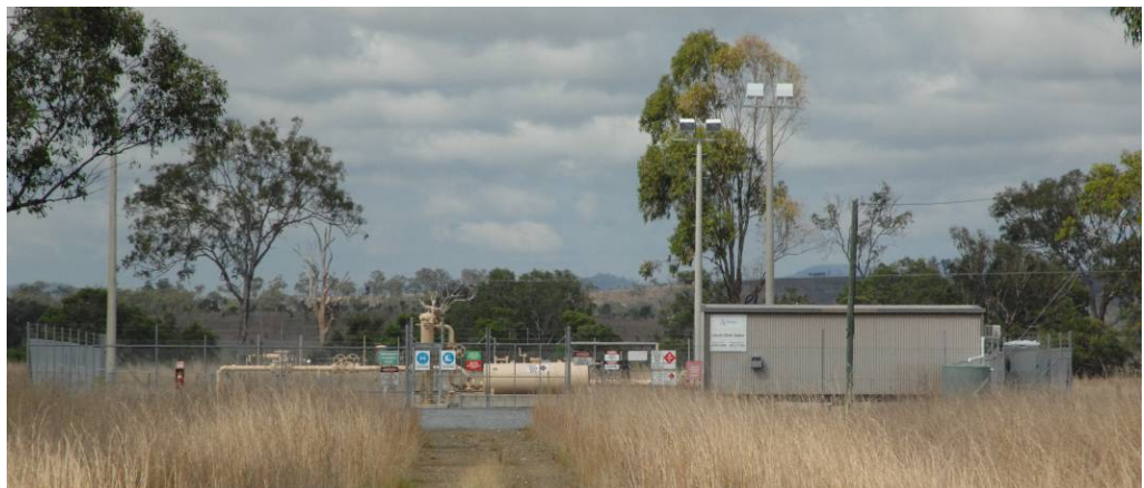
Figure 6.65 Larcom Creek Compressor Station (Alinta)
