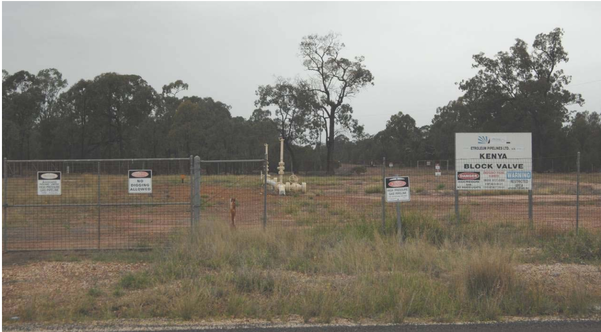
Figure 3.6 Illustrative view of a Mainline Valve
