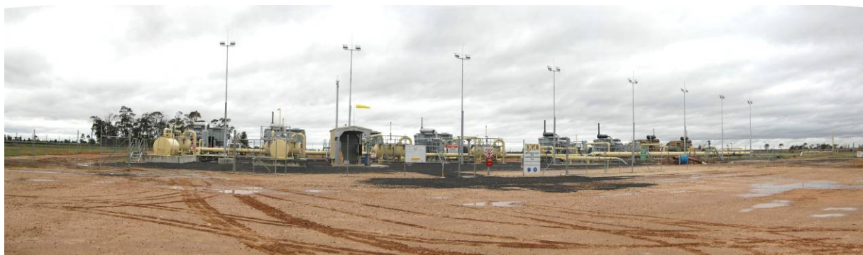
Figure 3.7 Illustrative view of a typical Field Compressor Station.
