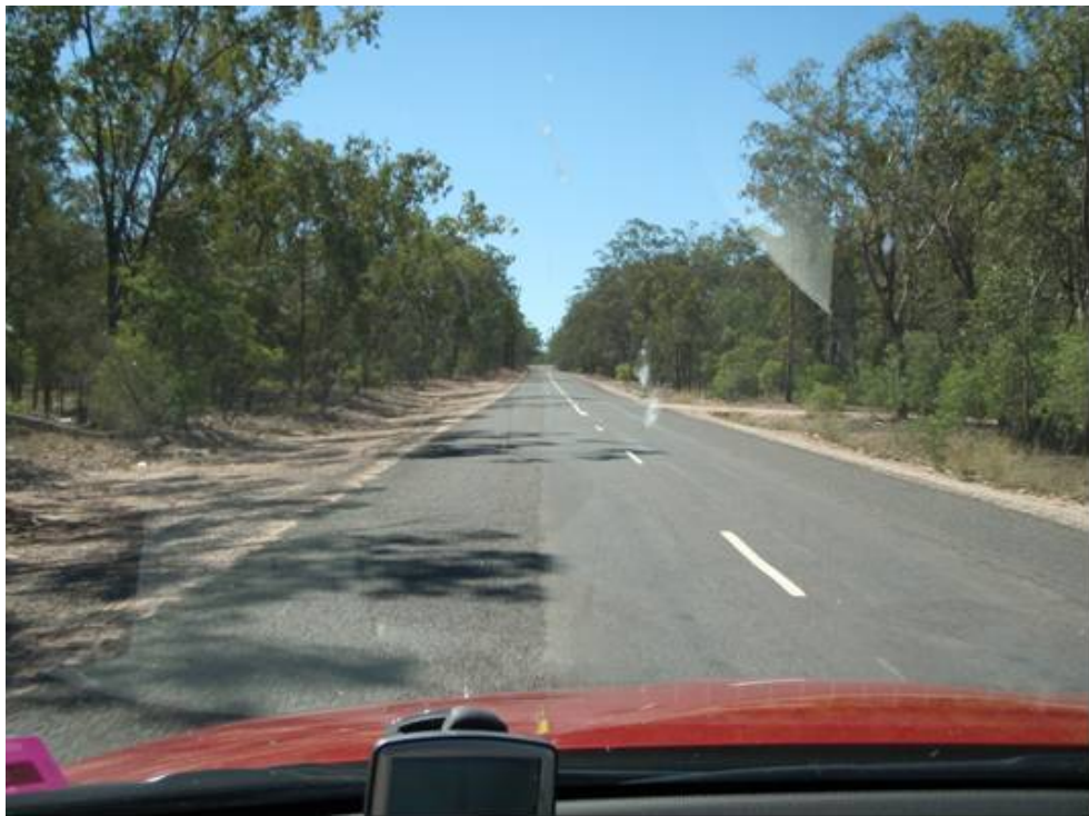
Figure 2.3 KOGAN-CONDAMINE ROAD—UNSEALED SHOULDERS
