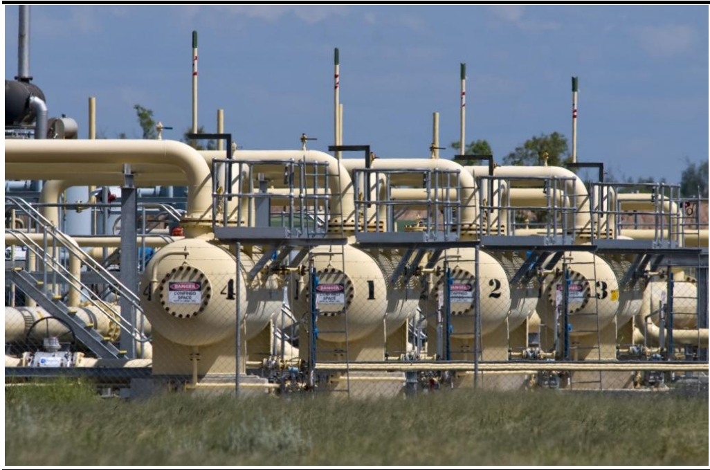
Plate 2.7.4 Section of a FCS showing Four Screw Compressors
