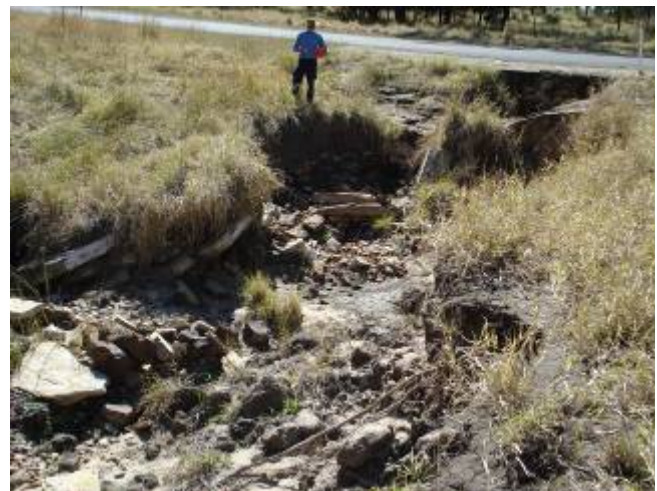
b) Erosion downstream of culvert
