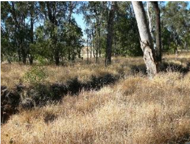
a) Eroded drain in the road reserve adjacent to Nathan Road
