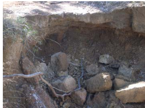
Photo: Undercutting Downstream Bank
