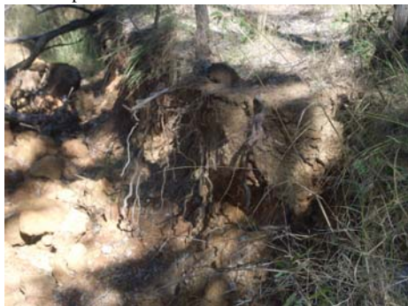
Photo: Eroded Downstream Bank
