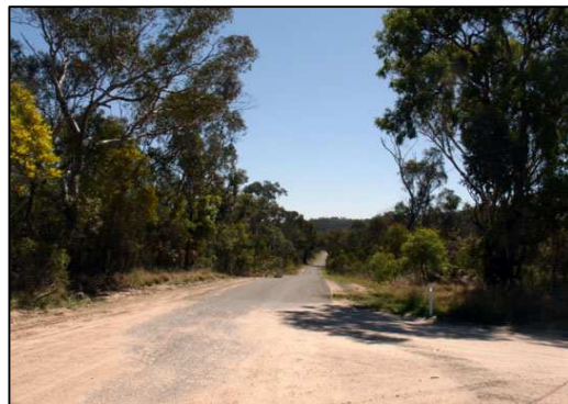
Figure 15: A common example of poor GSV along the road reserves.
