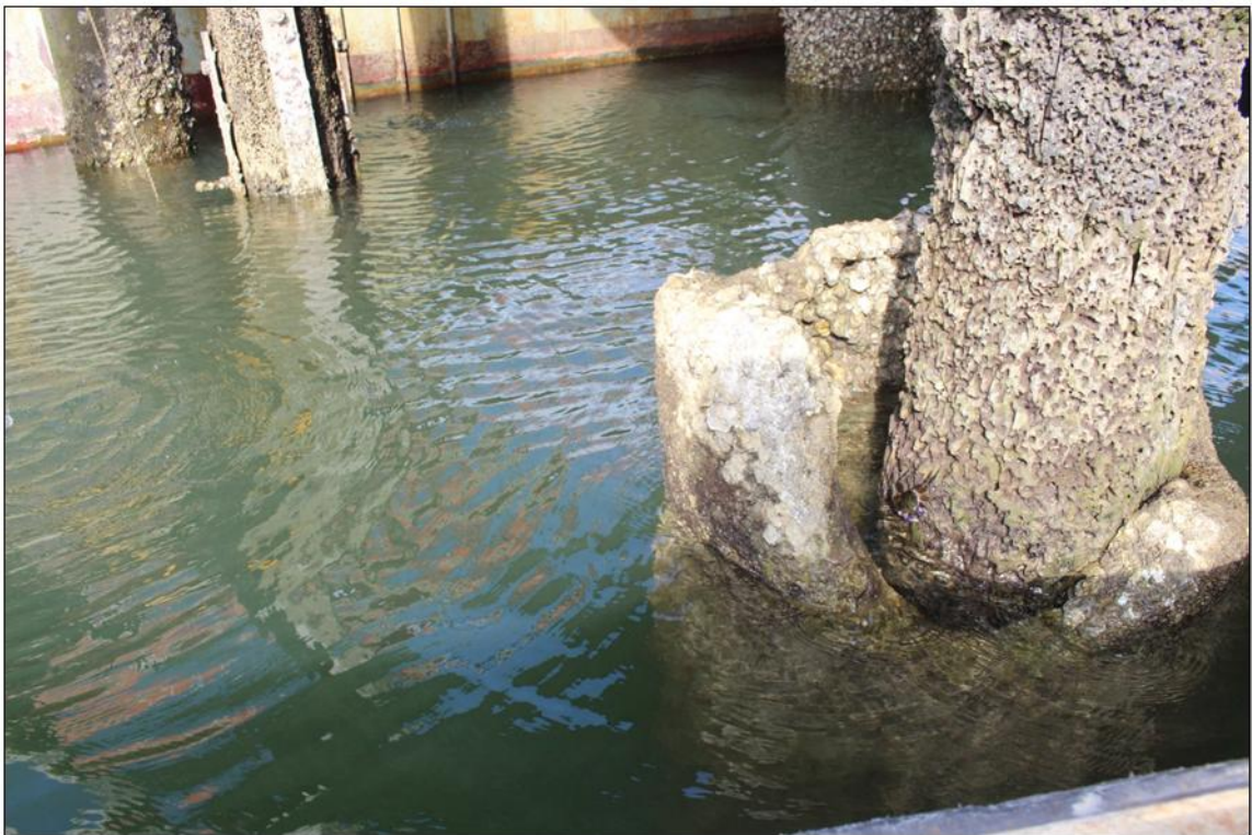
Damage to concrete sleeve.
