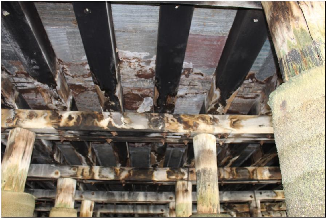
Staining to timber girders.
