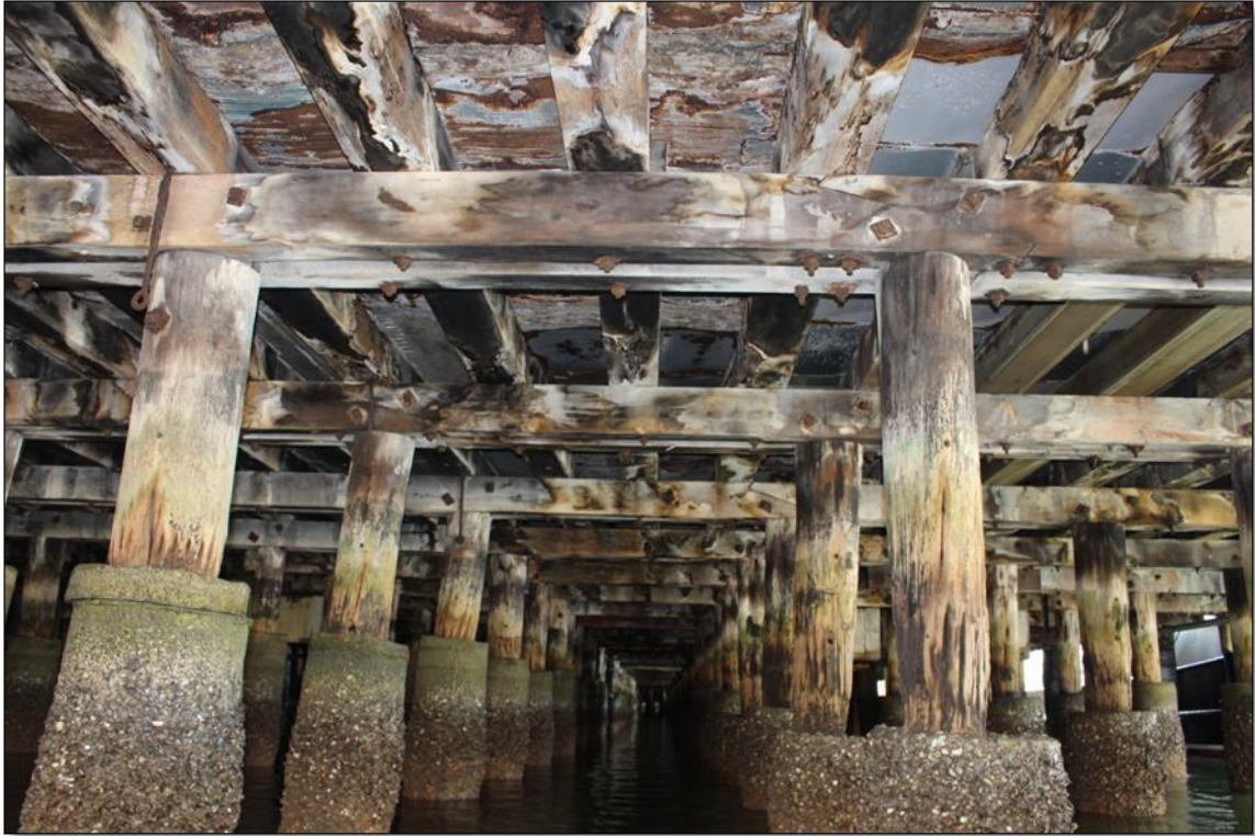
Degraded and decayed portion of piles visible above the concrete sleeves. Variable height of concrete sleeves.
