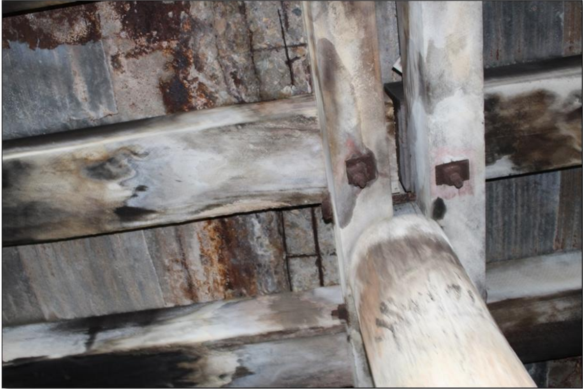
Corrosion to steel rods, nuts and washers.
