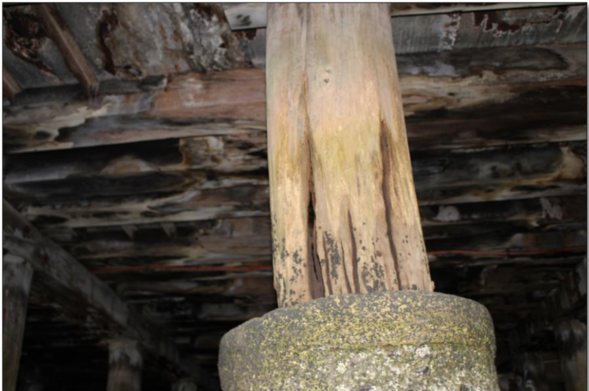
Splitting of pile.
