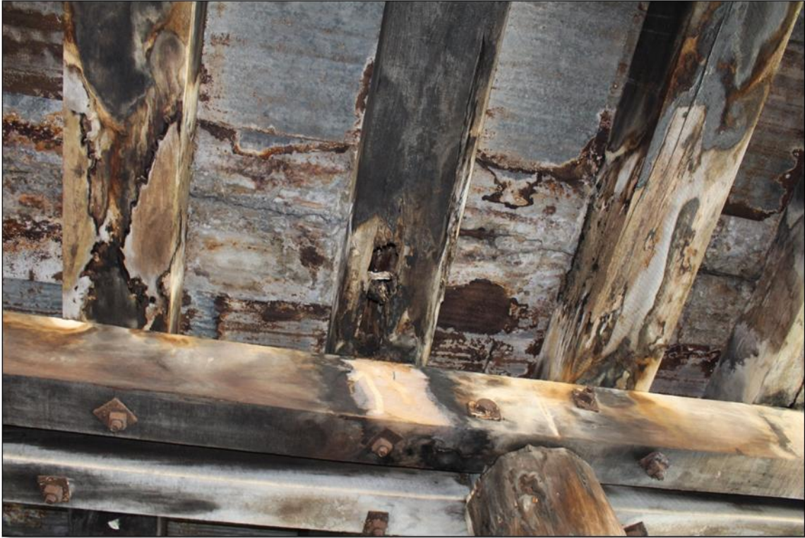
Advance degradation and decay to timber girders.
