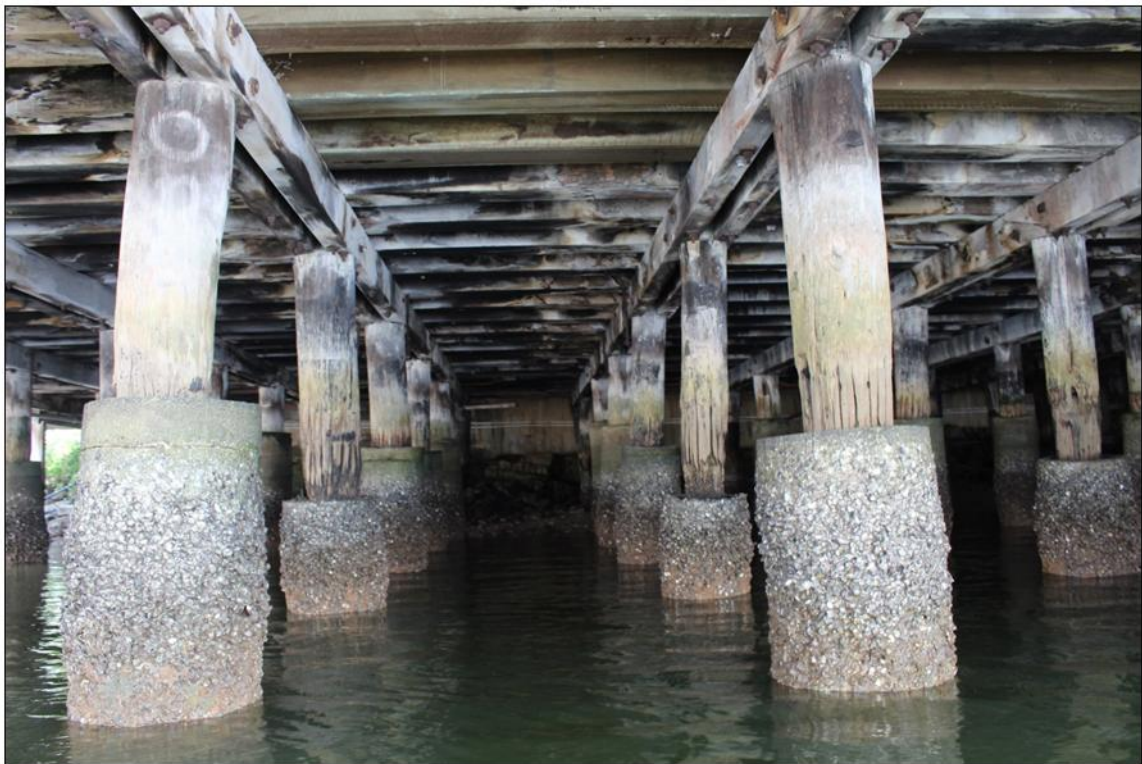
Degraded and decayed portion of piles visible above the concrete sleeves. Variable height of concrete sleeves.
