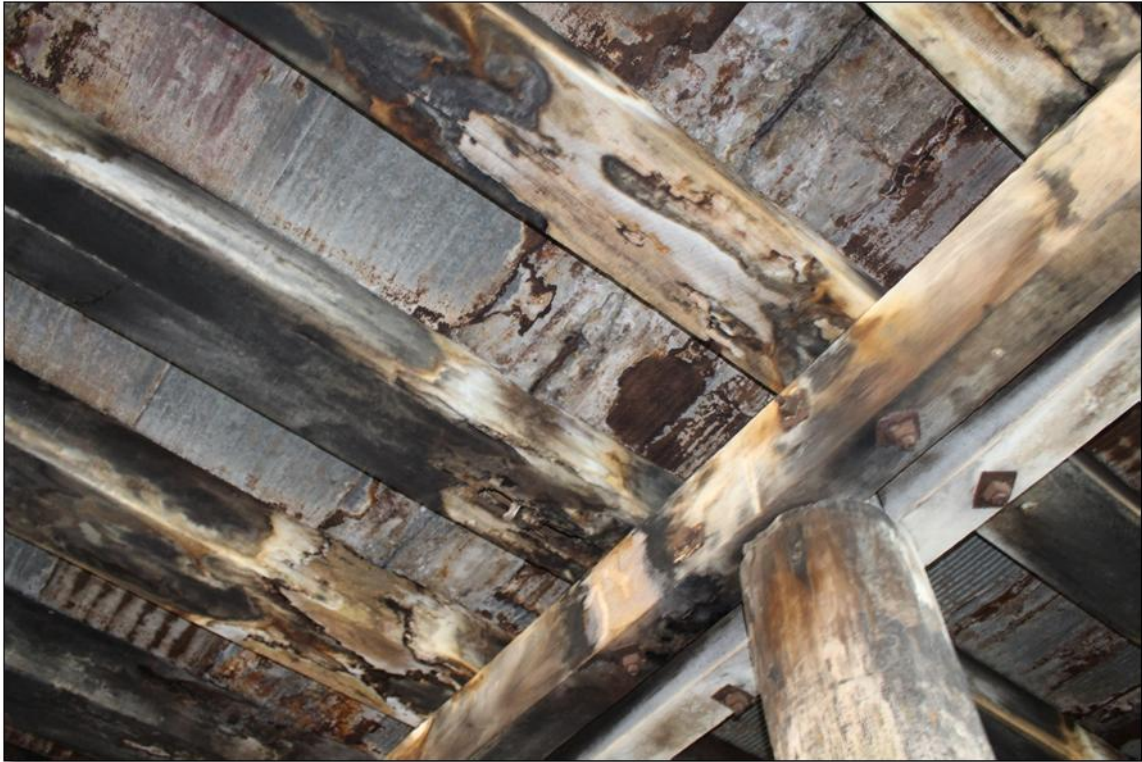
Staining and damage to timber
