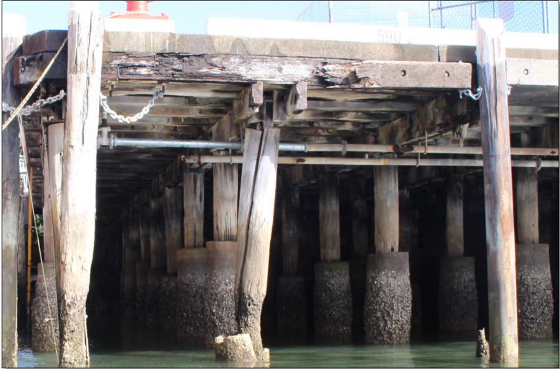
Splitting of pile and damage to concrete sleeve.
