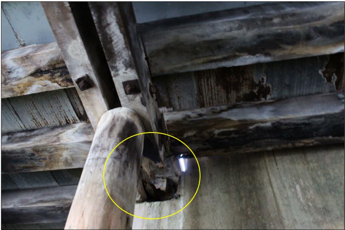
Localised damage to headstock.
