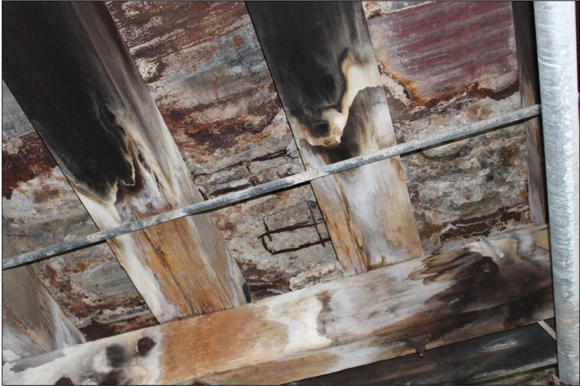
Corrosion to iron steel. Portions of the sheeting had completely rusted away.
