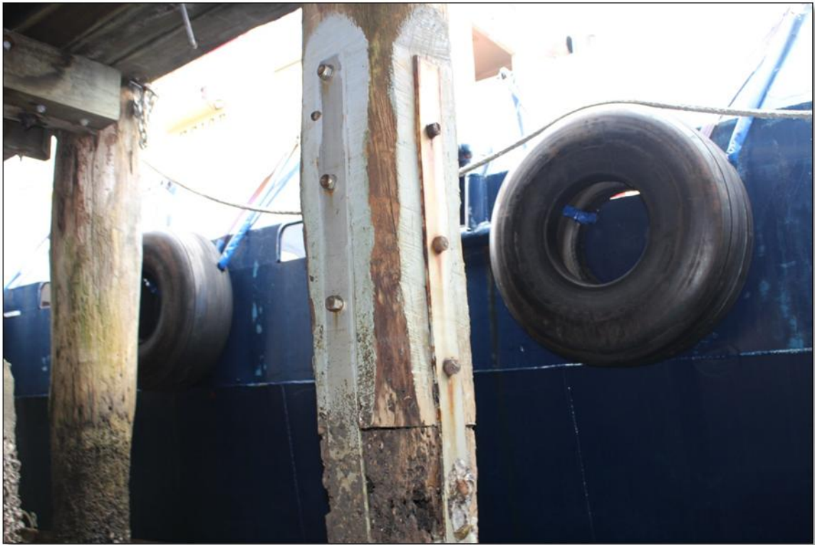
Spliced piles connected with steel plates bolted around the perimeter of the pile
