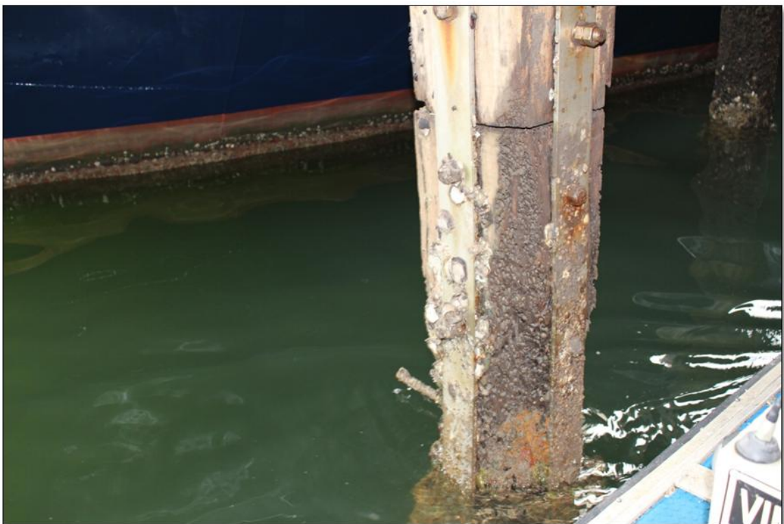
Spliced piles connected with steel plates bolted around the perimeter of the pile
