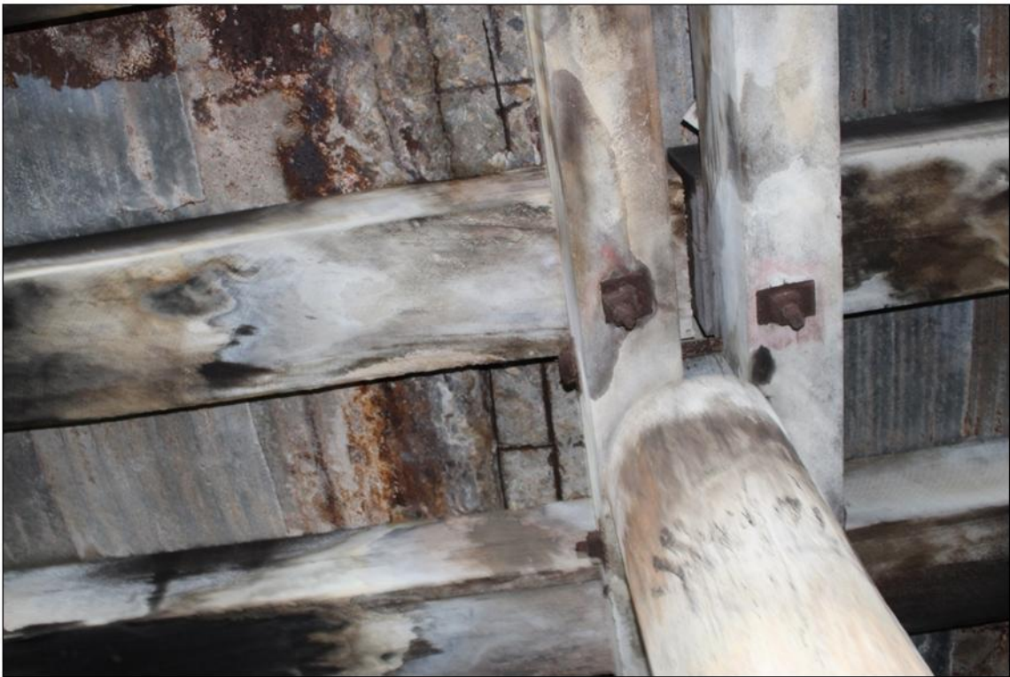
Severe corrosion of bottom reinforcement. Steel sheeting to underside of deck has completely rusted away.
