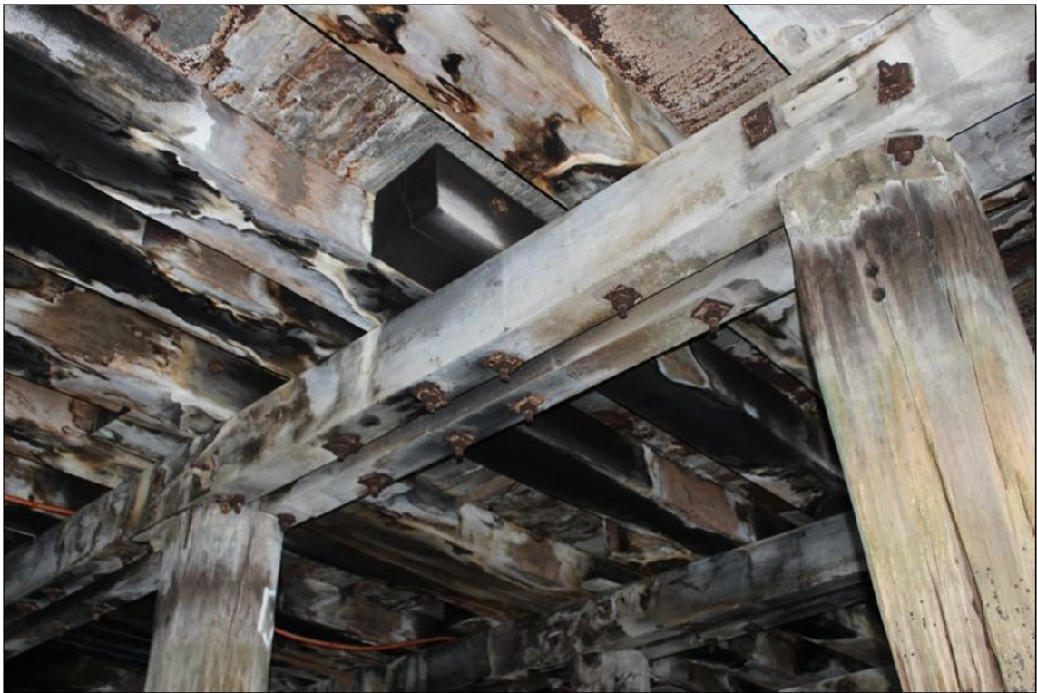
Corrosion to steel rods, nuts and washers.
