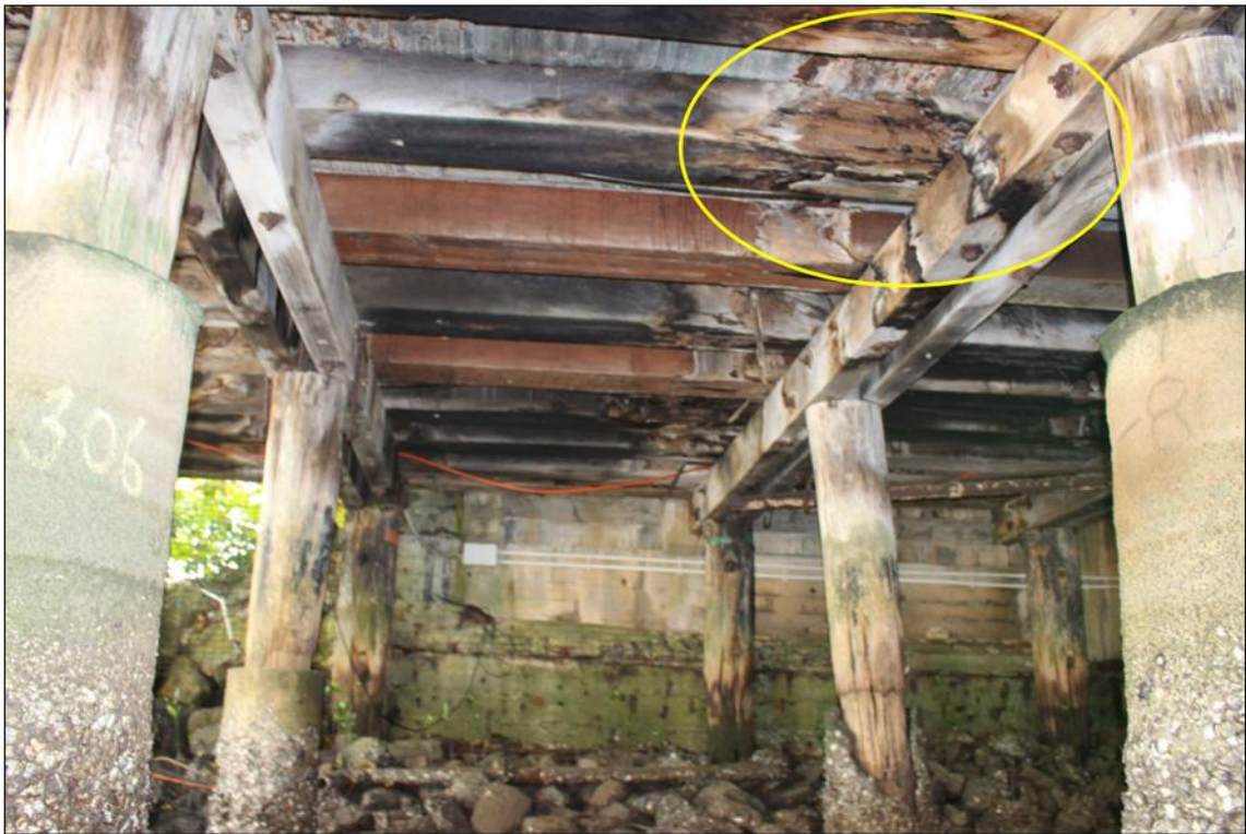
Advance degradation and decay to timber girders.
