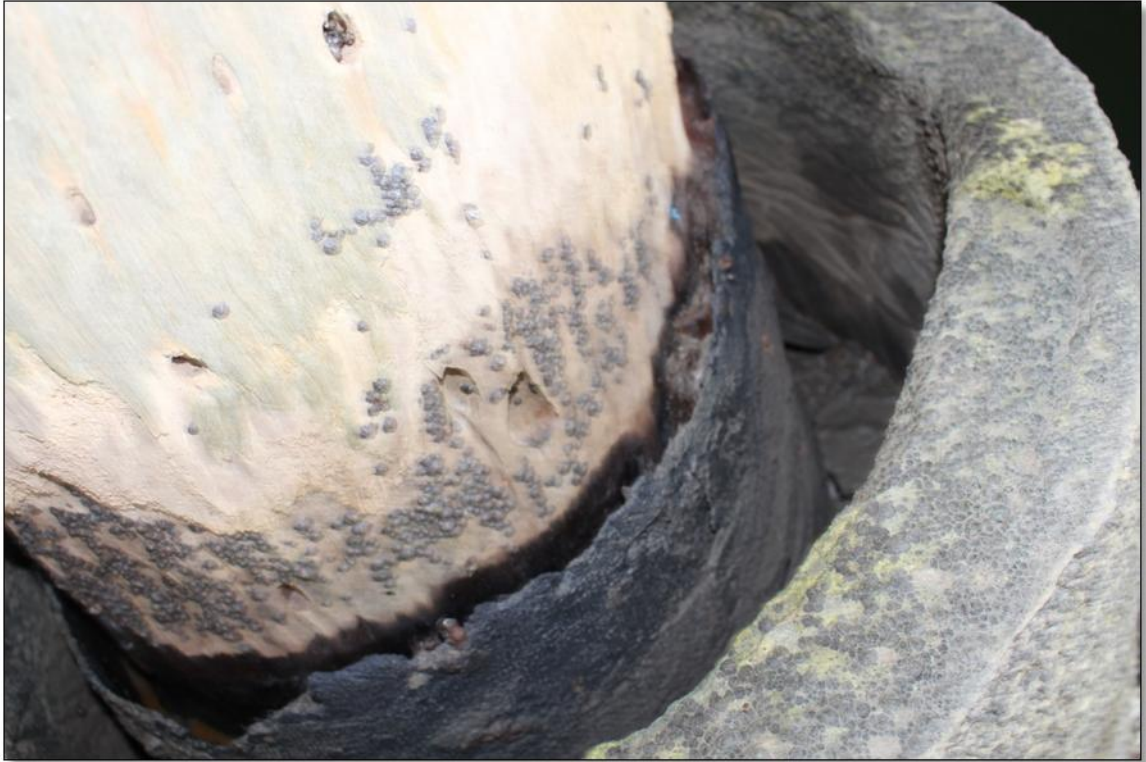
Void between the pile and the concrete sleeve.
