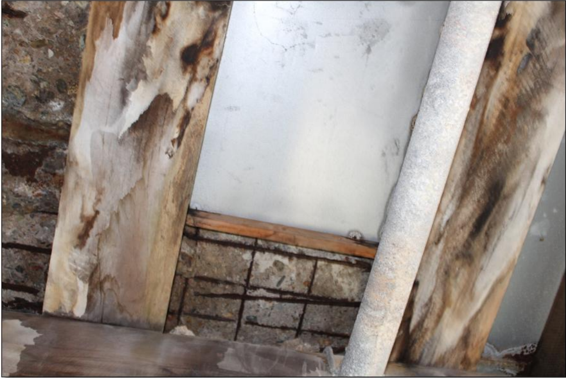
Severe corrosion to bottom reinforcement. Steel sheeting to underside of deck has completely rusted away.
