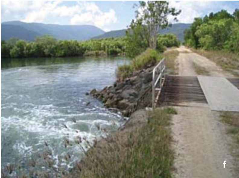
Figure B13.8f-h Bund Wall at Hills Creek with flow gates. View to ENE
