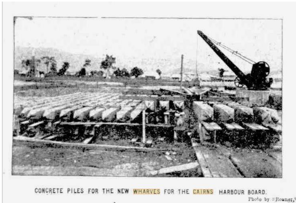
Figure 12. Photograph of the Concrete Piles for the Cairns Harbour Board, published in 'The Week', Friday, 30 December, 1910. (Source: Trove)
