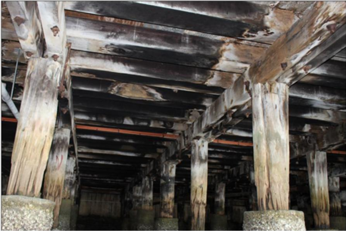
Figure 29. Image of the deteriorating piles and structure at Wharf 6 (from Appendix AE Condition Assessment).
