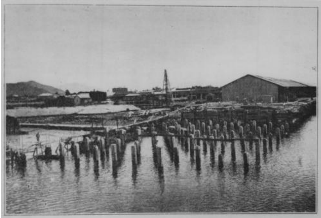
Figure 15. New section of reinforced concrete wharf (Wharf 5) under construction at Cairns, circa 1923. (Source: SLQ #199171)
