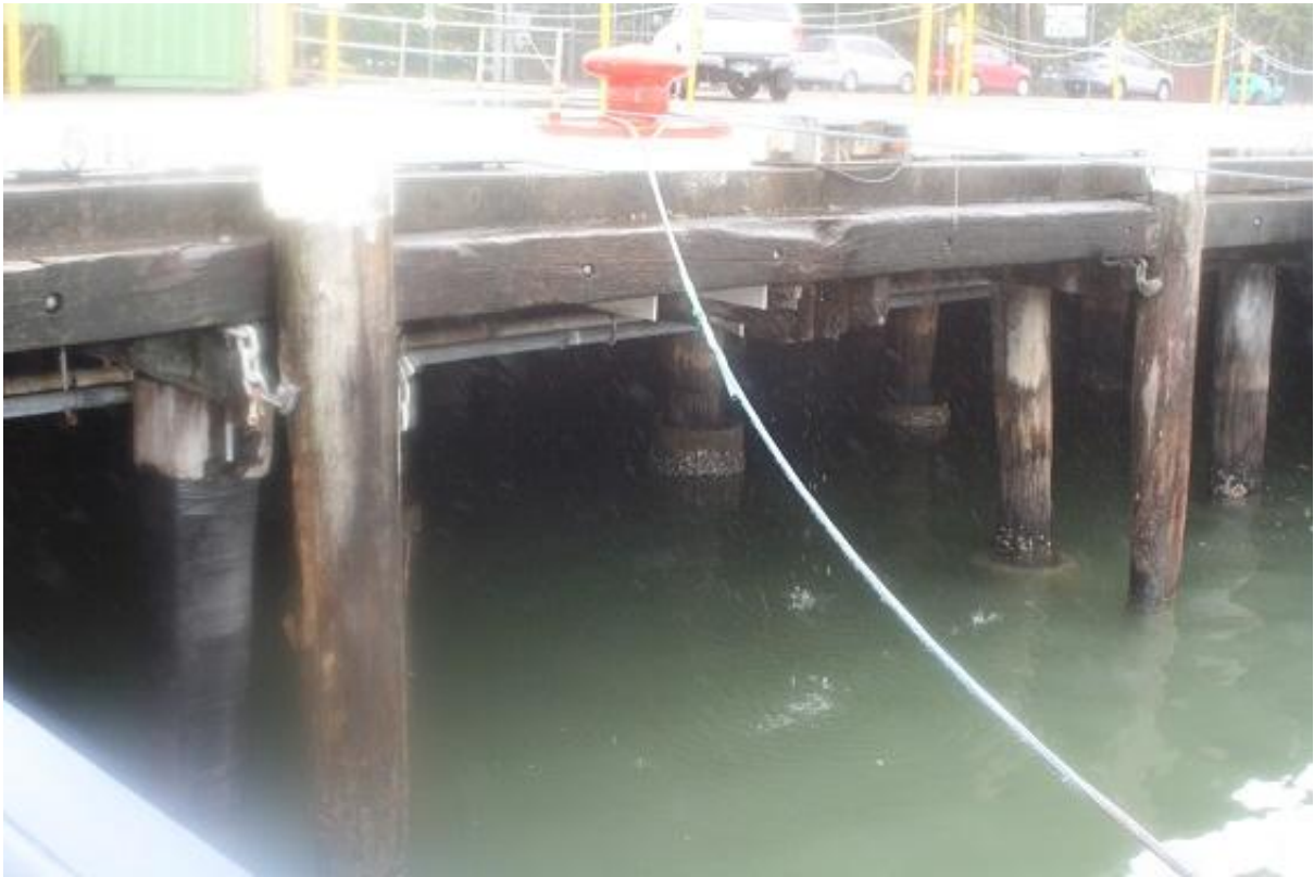
Figure 22. The timber substructure of Wharf 6 is in poor condition.
