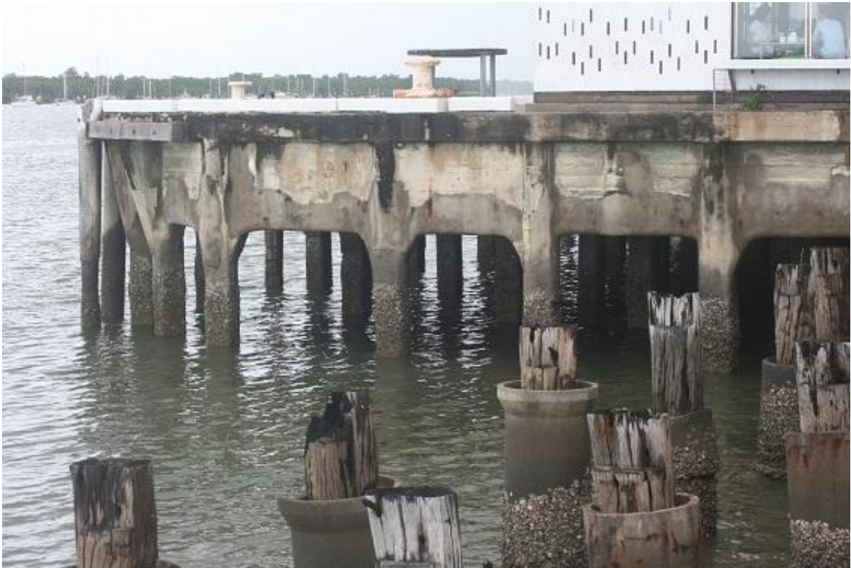
Figure 20. The reinforced concrete structure is apparent at the north end of Wharf 1.
