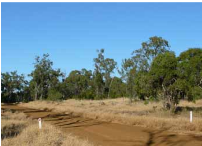
Plate 9-3. A narrow, single lane, formed earth, section of Nathan Road between Cockatoo Creek and Maidens Road
