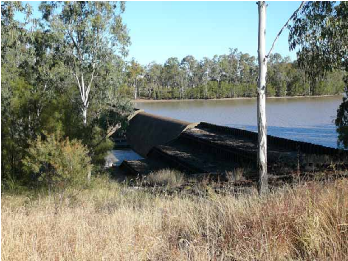
Plate 1-1. Glebe Weir showing central spillway flanked by stepped rows of steel sheet piling and with stilling pond downstream of the spillway.
