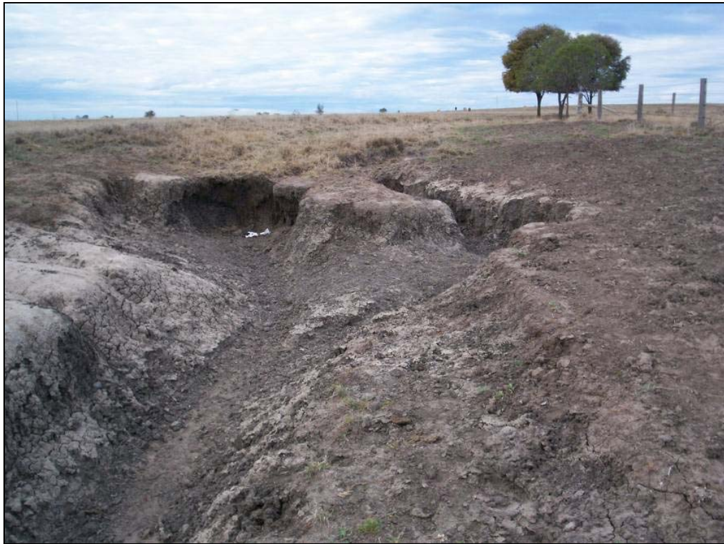
Photo 9-1: Gullyhead erosion caused by exposure of dispersive soils in a drainage line on a gentle slope near WS26
