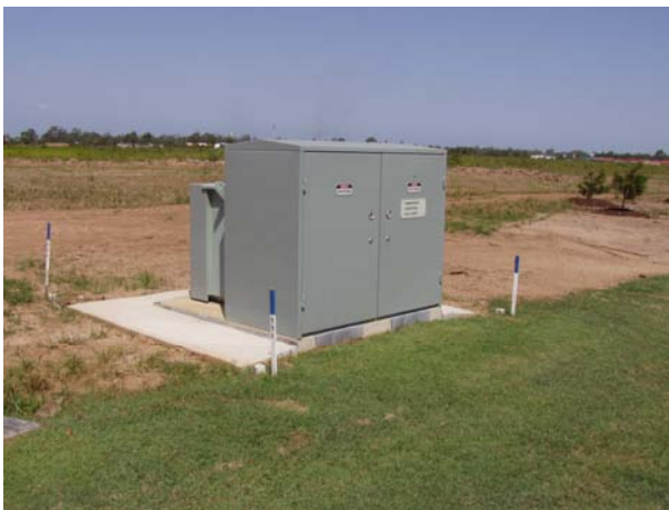
Photo 7: Example of a Padmount Transformer (PMT).
