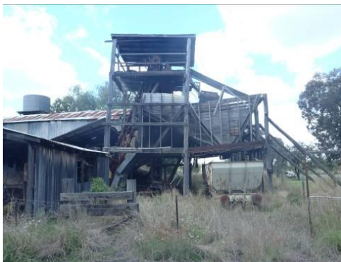
Photograph 12-1 Gantry and Hopper
