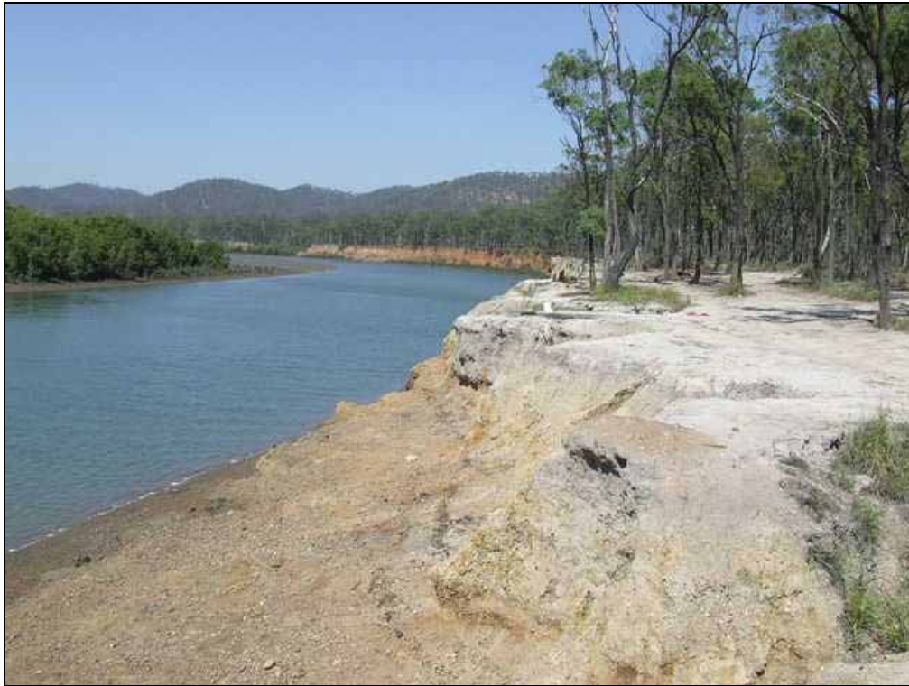
Figure 9 Eroded bank – looking south west along the oxbow of the Calliope River
