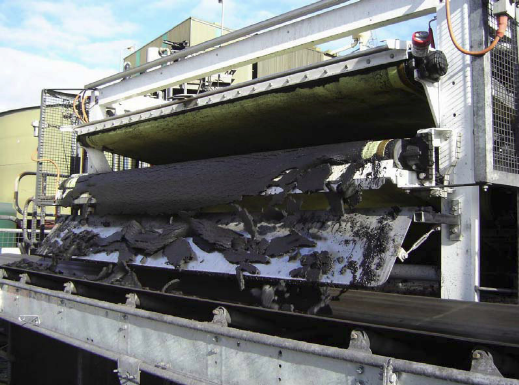
Figure 4 Belt press filter in operation in a Hunter Valley coal mine operation
