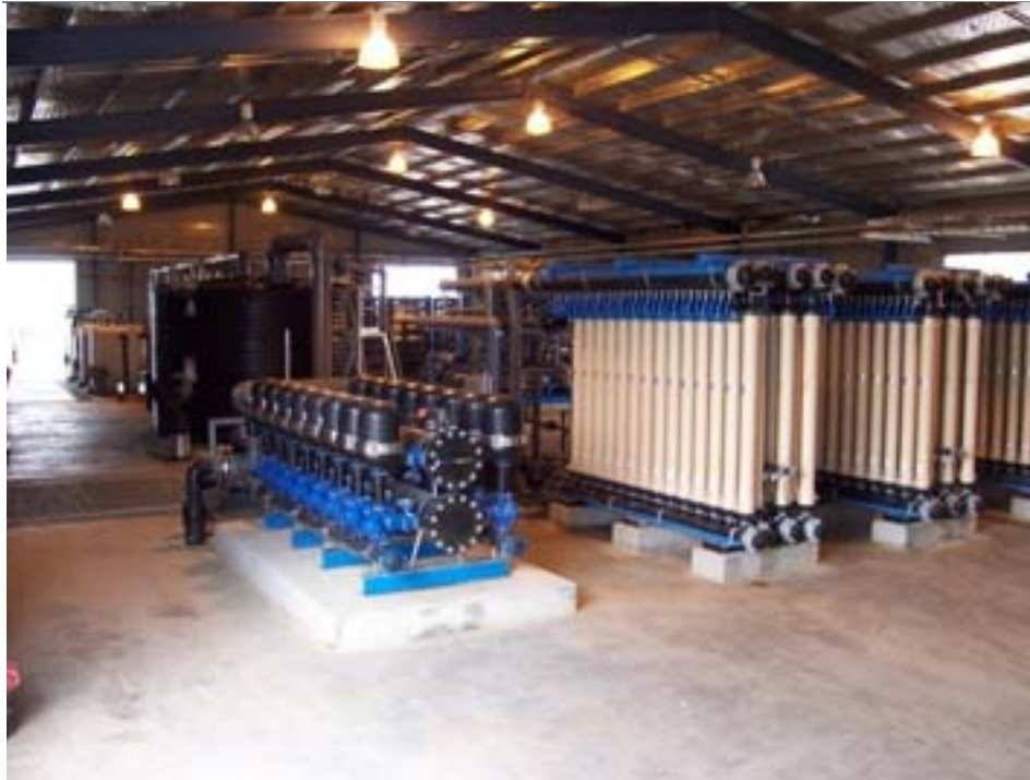
Plate 6.2 Membrane filtration system at Spring Gully WTF
